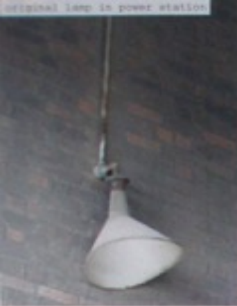
lamp in power station
